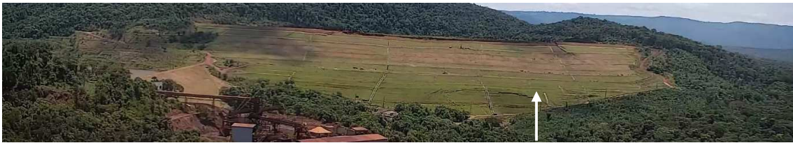
Figure 6: Bulging Above the Toe of the Dam Approximately One-Third in from the Left Abutment (Right Side of Photograph), Initiated About 0.2 s After the First Observed Deformation at Crest
