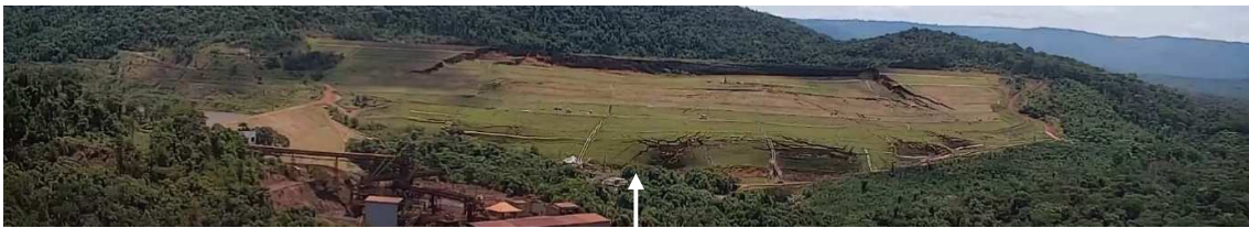
Figure 7: Continued Settlement of the Crest and Bulging Above the Toe with Water Erupting Above the Toe Toward the Right Abutment (Left Side of Photograph) About 5.5 s After the First Observed Deformation at Crest
